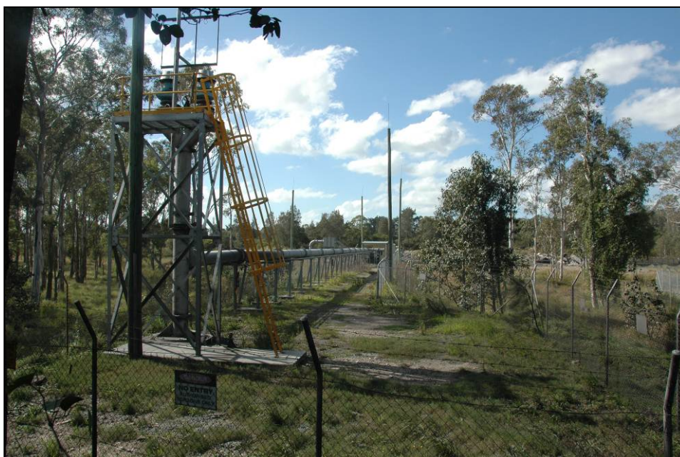
Plate 1 – Methane gas drainage pipeline and ventilation stack at Mandalong
