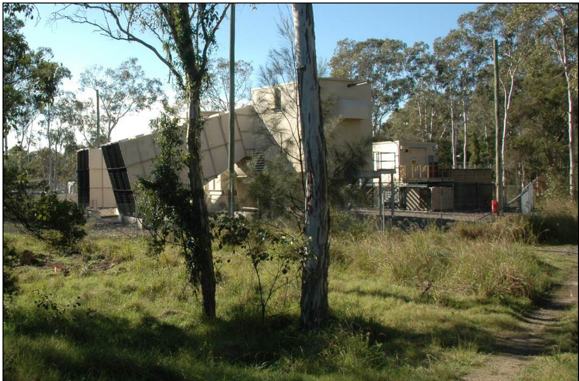
Plate 2 – Main mine ventilation fans
